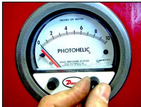
Fig. 11 – Automatic Damper Maximum Closed Setting
